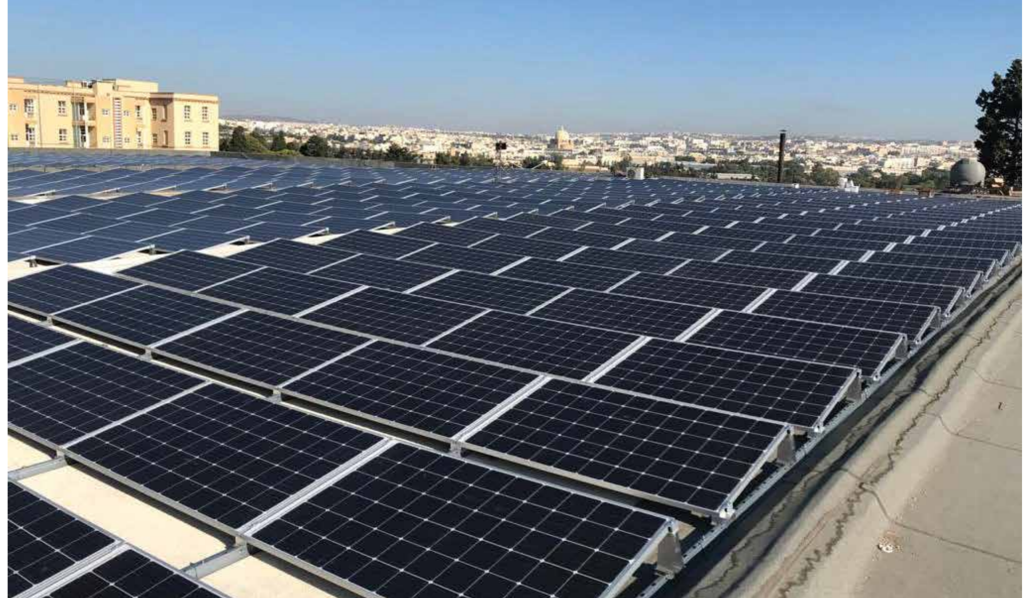
Nexos Manufacturing , Marsa 245.52 KWp 792 PV Modules
