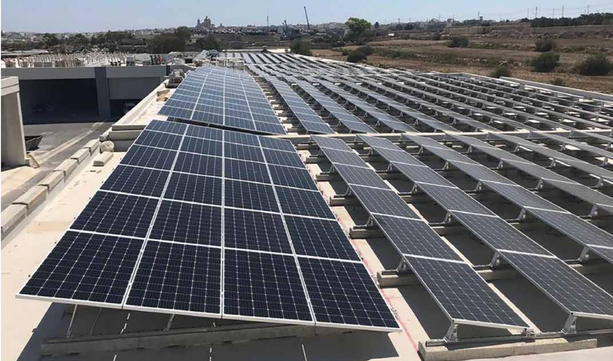
Faizon Industrial Complex , Ghaxaq 600 KWp 2000 PV Modules
